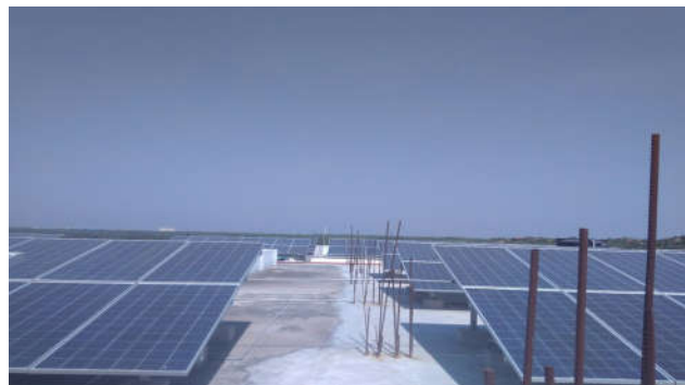
Fig .4 Actual onsite of 80KW solar roof top plant at St.Peter’s Engineering College, Hyderabad City
