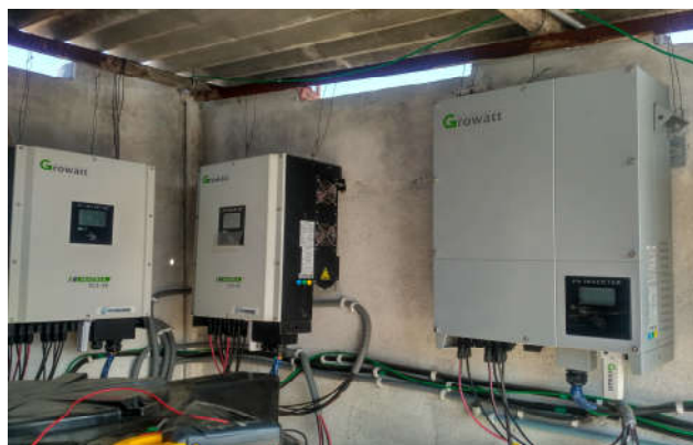
Fig.6 Actual onsite 80KVA solar grid inverter at St.Peter’s Engineering College, Hyderabad City
